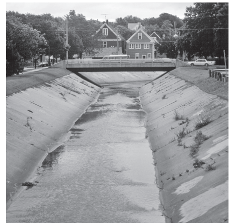
Note the presence of any artificial embankments. This stream has a fortified concrete embankment.
